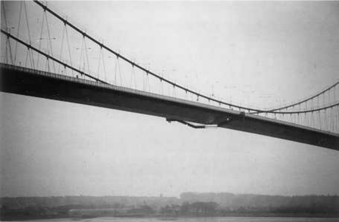
Figure 1 Humber Bridge midspan with targets for optical deflection tracking
