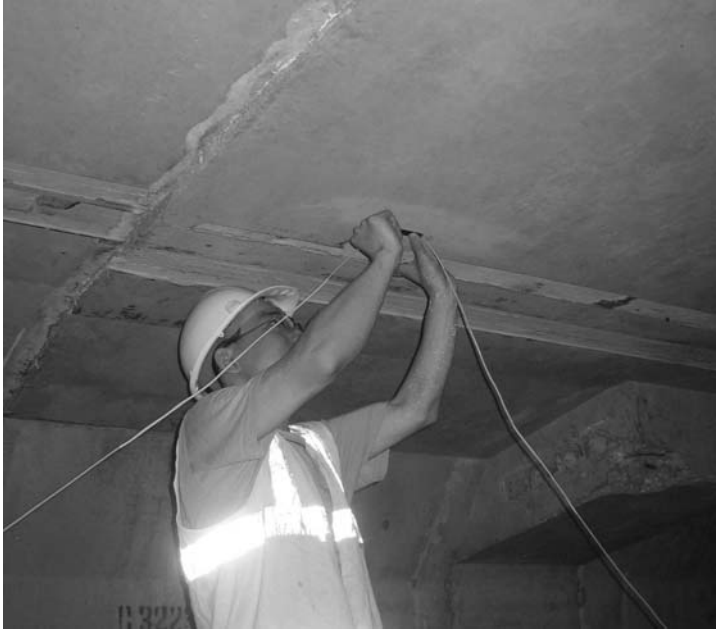
Figure 18 Inside box deck for mounting FBGs
